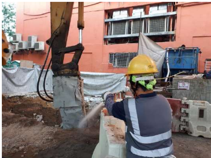
Figure A1 Noise barrier mat fully covered for the breaker's head and water spraying during breaking
